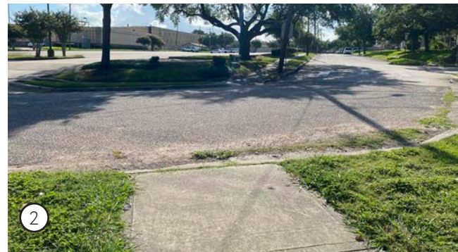
Neighborhood park entry that does not meet ADA accessibility requirements due to change in elevation
