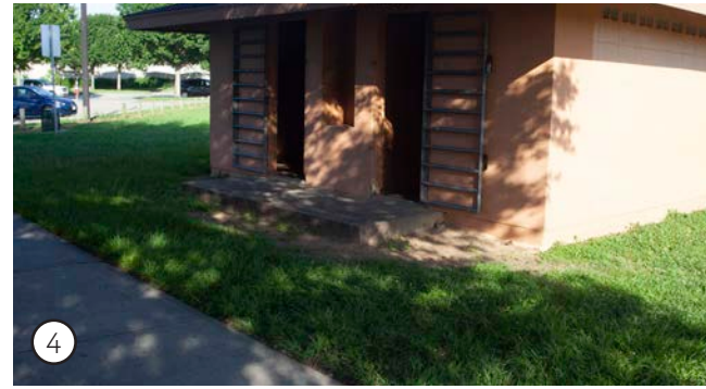
Rest room that is inaccessible due to lack of ramp and path connection
