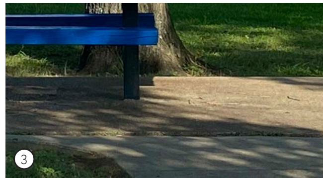
Path to picnic area that does not meet ADA accessibility requirements due to change in elevation
